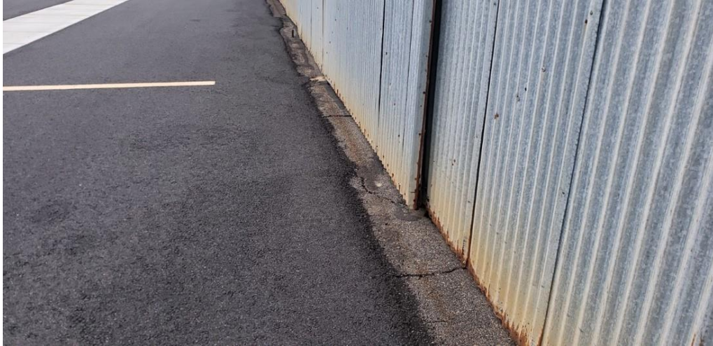
Hangar Floor Transition Area Problem; Photo: Jury Member
