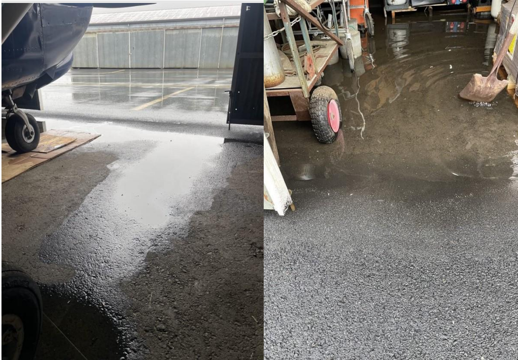
Pooling water problem in one of the Columbia Airport Hangars; Photo: Jury Member
